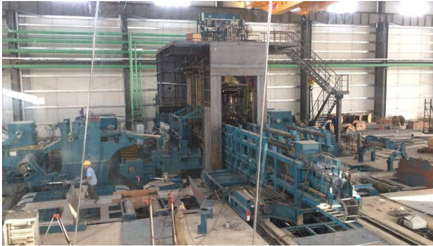
Picture 2 : installation of the single stand 6-high reversing cold mil at workshop No.4 (phase 2)
